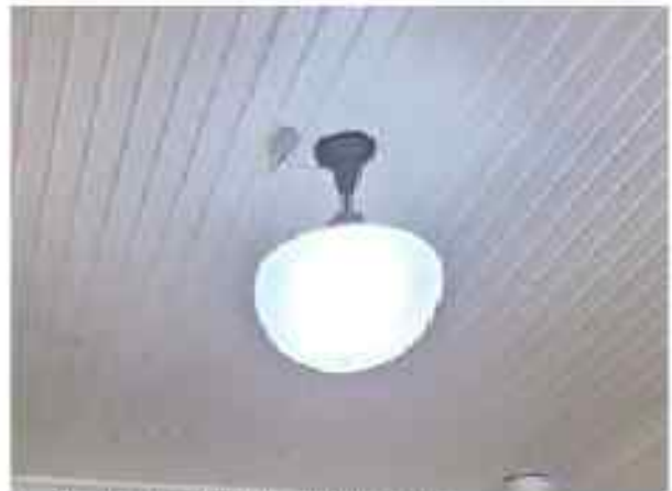
Image 106 – Typical pendant at 3rd Floor Corridor
