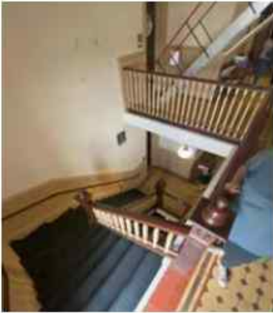
Image 139 - Lighting levels in the stairwell are not sufficient.
