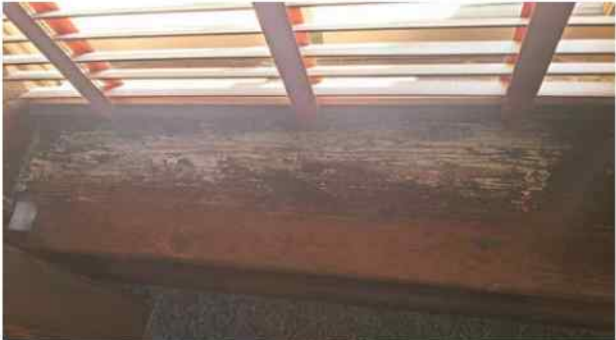
Image 58 - Typical wood deterioration at District Courtroom Windows
