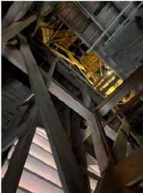
Image 134 - Interior of central tower wood framing with isolated regions of water accumulation.
