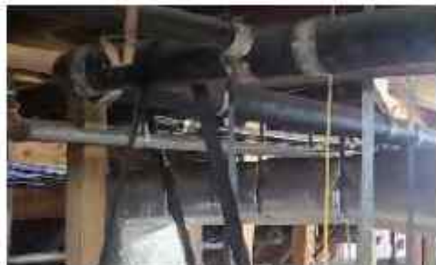
Image 143 - Overhead cat-in-the-hat piping in attic
