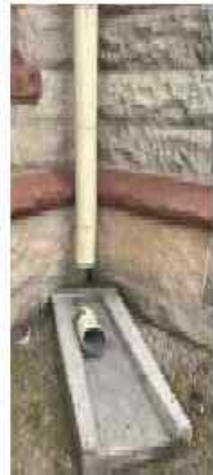
Image 51 - Damaged downspout on West Elevation
