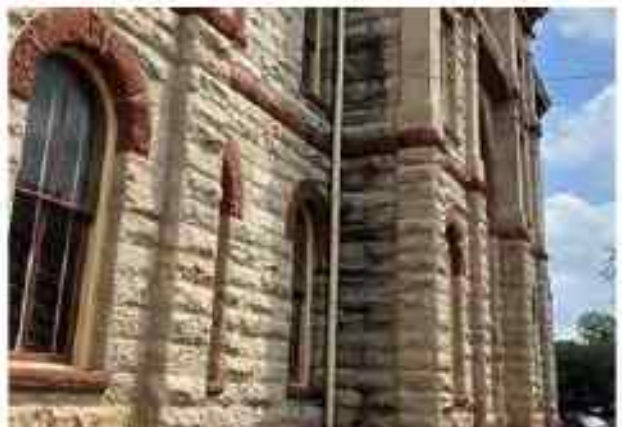
Image 129 - Example of biological growth on east facade
