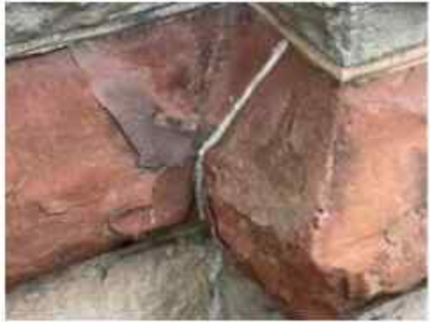
Image 127 - Example of delamination in sandstone
