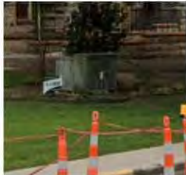
Image 44 - Transformer boxes at the northeast corner of the site.
