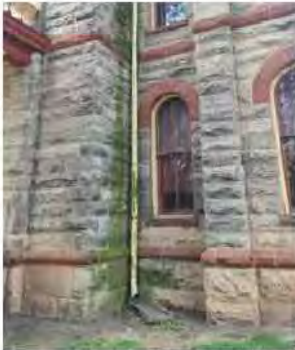
Image 53 - Biological growth on exterior wall
