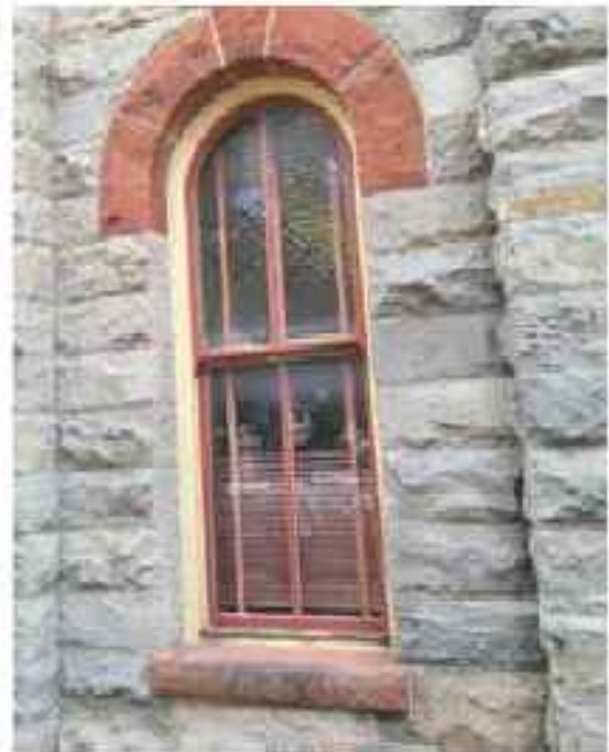
Image 62 - First floor window at north elevation with severely damaged wood sill.
