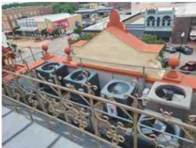
Image 4 - View of rooftop mechanical unit from main roof.
