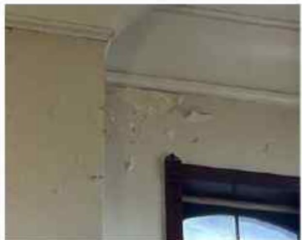
Image 131 - Example of peeling paint within Coit room
