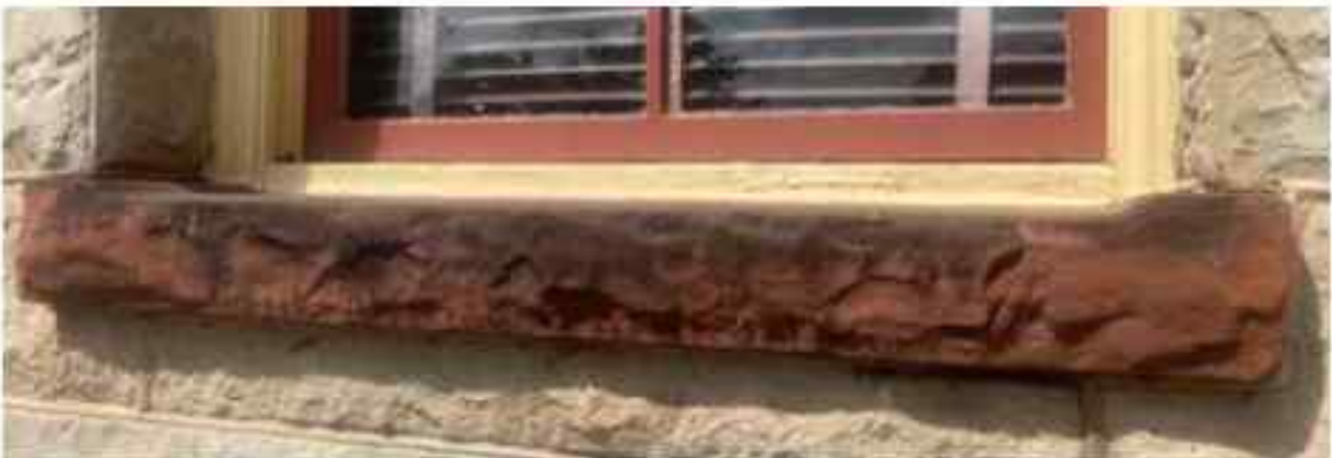
Image 63 - Peeling paint & black staining at rear window
