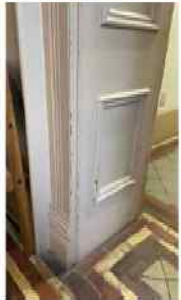
Image 95 – Typical damage to door casing
