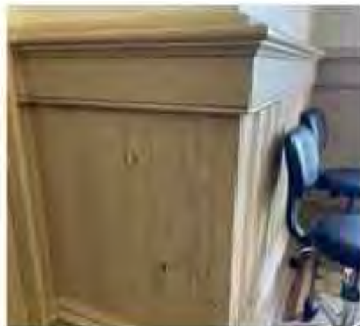
Image 84 – Damaged wood wainscoting
