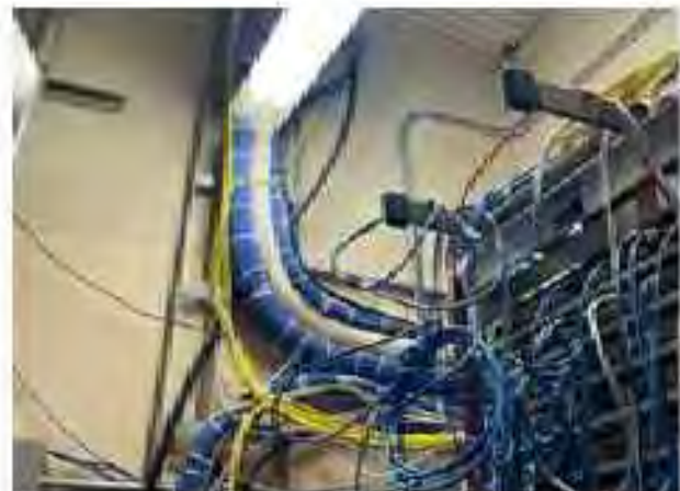
Image 3.68 – IT Closet infrastructure on second floor
