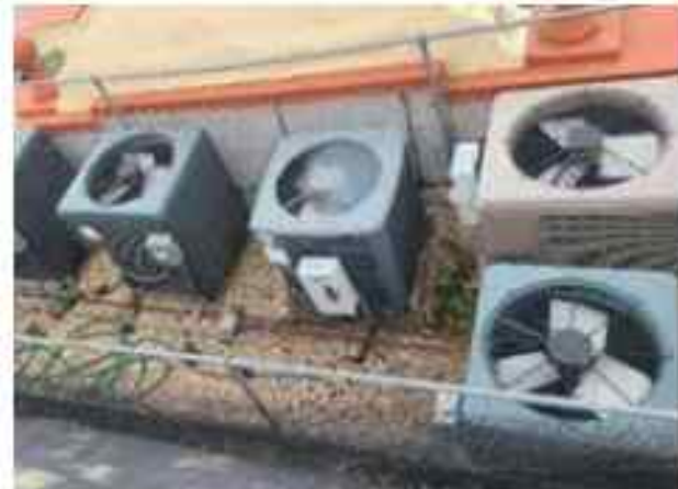
Image 135 - Conditioning units within "mechanical terrace" on low roof.
