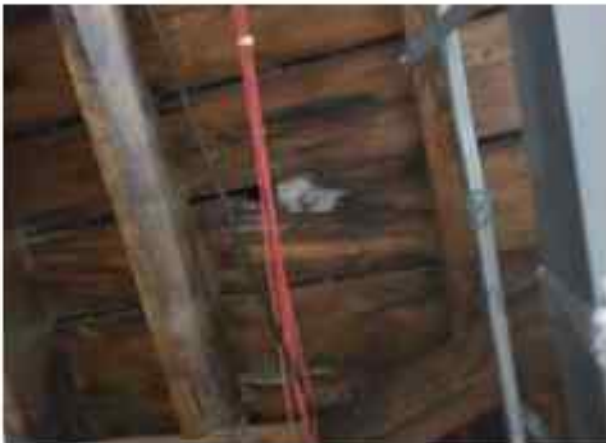
Image 111 - Damage at roof deck in attic.
