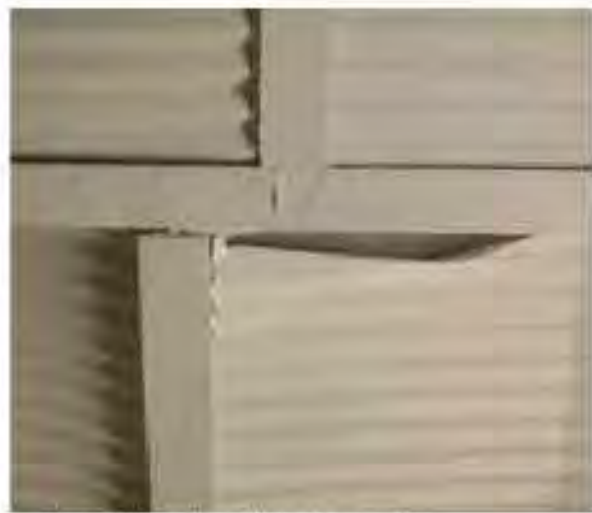
Image 78 - Paint peeling on 1st Floor Main Corridor
