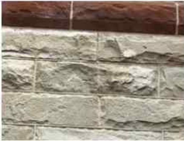
Image 126 - Example of cracking in limestone
