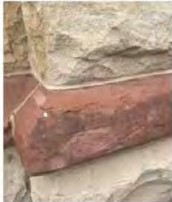
Image 54 - Typical cracking/spalling of Pecos sandstone
