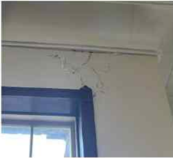
Image 132 - Recent plaster cracking above window in Courtyard.
