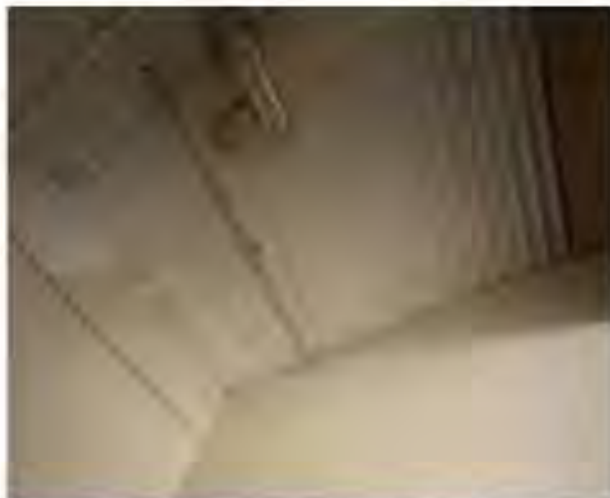
Image 144 - Unsealed pipe penetrations in 2nd floor fire stair
