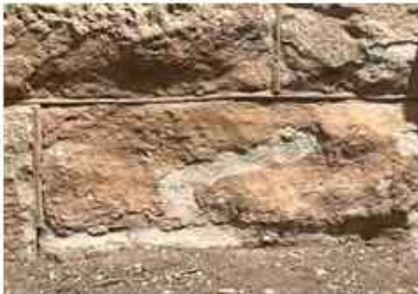
Image 128 - Example of delamination in limestone
