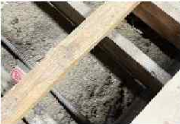
Image 109 - Commercial insulation in attic.
