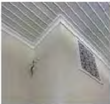
Image 83 – Peeling paint on plaster wall, third floor office / 911
