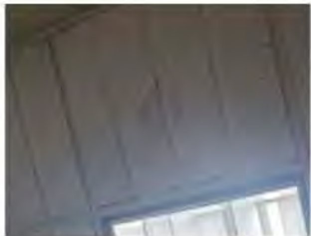
Image 80 - Women's restroom ceiling on 3rd Floor with typical water damage
