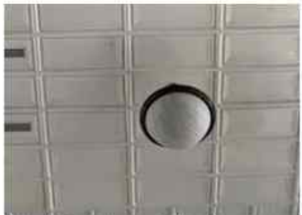
Image 105 – Typical non-historic pendant at Theater Courtyard
