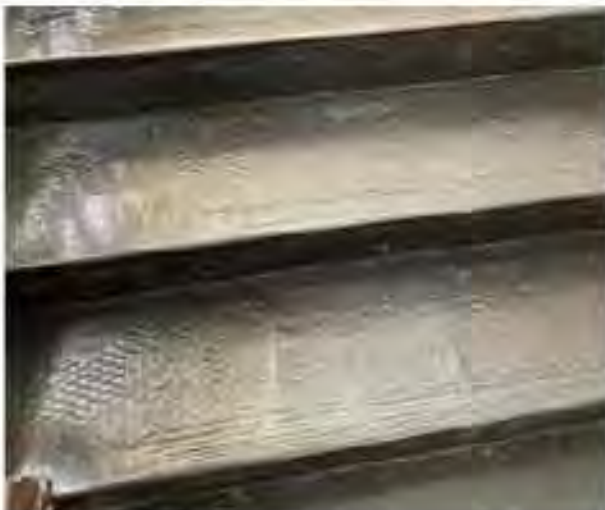
Image 85 - Sign of wear on the grand stair tread
