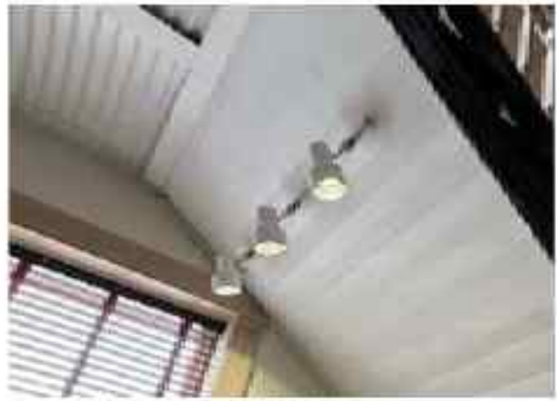
Image 102 – Track lighting at 2nd Floor Main Stairs
