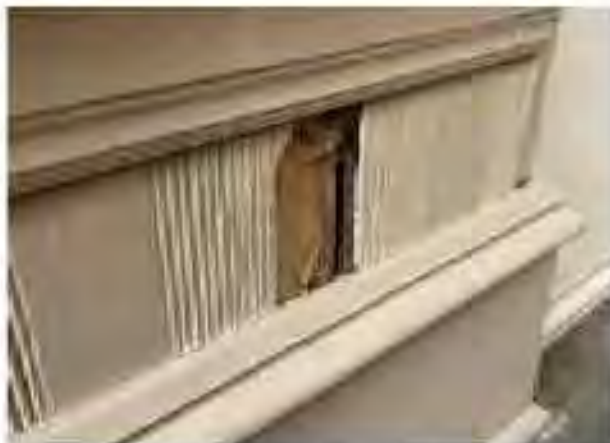
Image 112 – Damaged wainscot in First Floor Hallway 104
