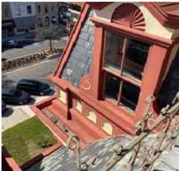
Image 45 - Main roofing at the main mansard and corner pavilion appears to have been partially coated in a paint or similar material.
