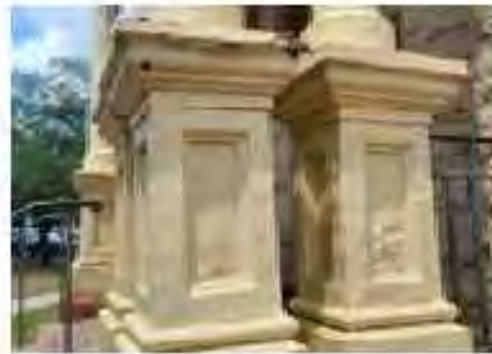
Image 66 - Distorted sheet metal on porch columns
