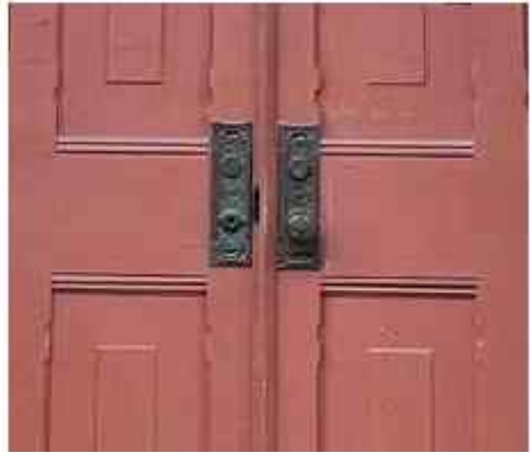
Image 60 - Exterior hardware are at non-ADA entries
