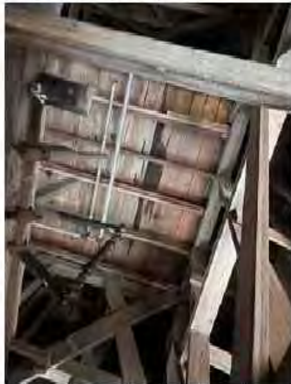
Image 50 - Example of water intrusion at principal tower attic space
