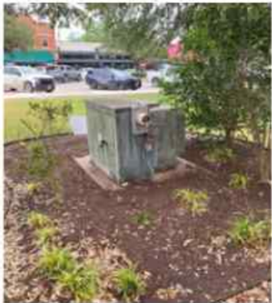
Image 140 - Electrical utility pad around perimeter
