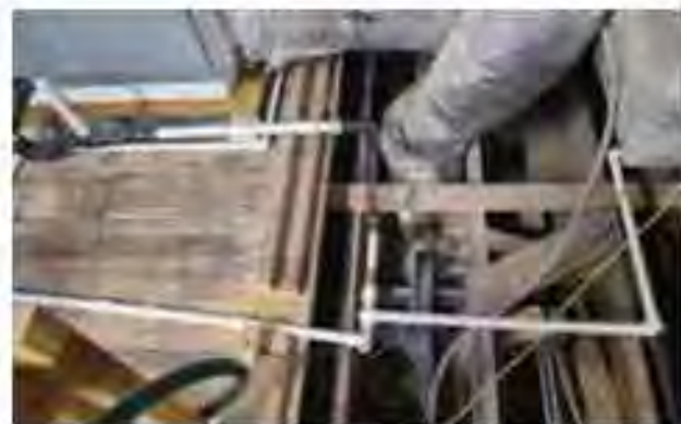
Image 138 – Condensate piping around the
