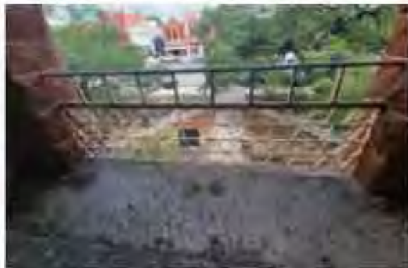
Image 68 - Second floor balcony off courtroom shows visible bird debris
