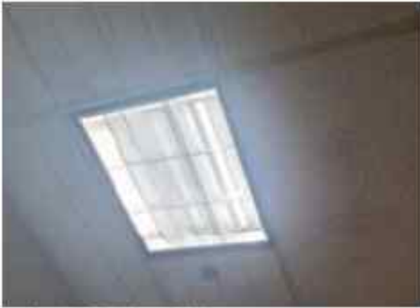
Image 101 – Typical aggregate light fixture in restroom
