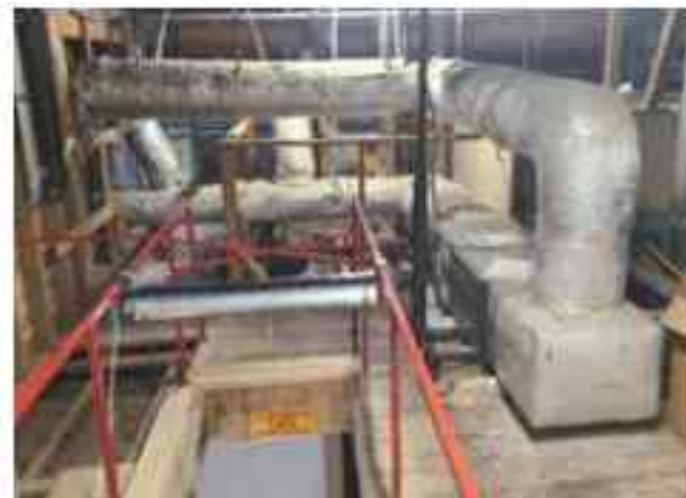
Image 136 - Supply/Return ductwork without balancing dampers.
