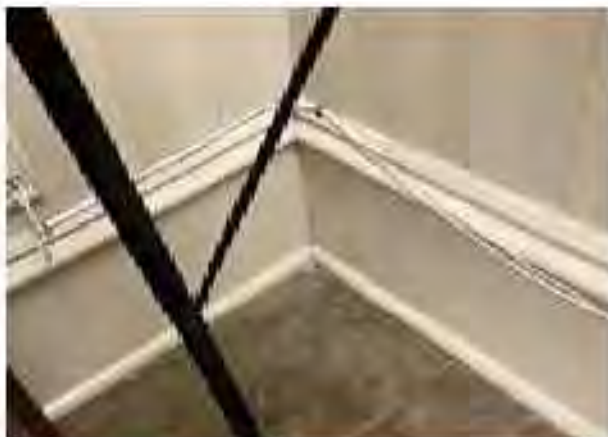
Image 3.67 – Surface mounted ethernet and/or telephone cabling in restrooms
