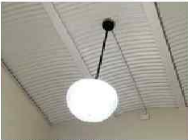
Image 103 – Typical pendant at 1st Floor Corridor
