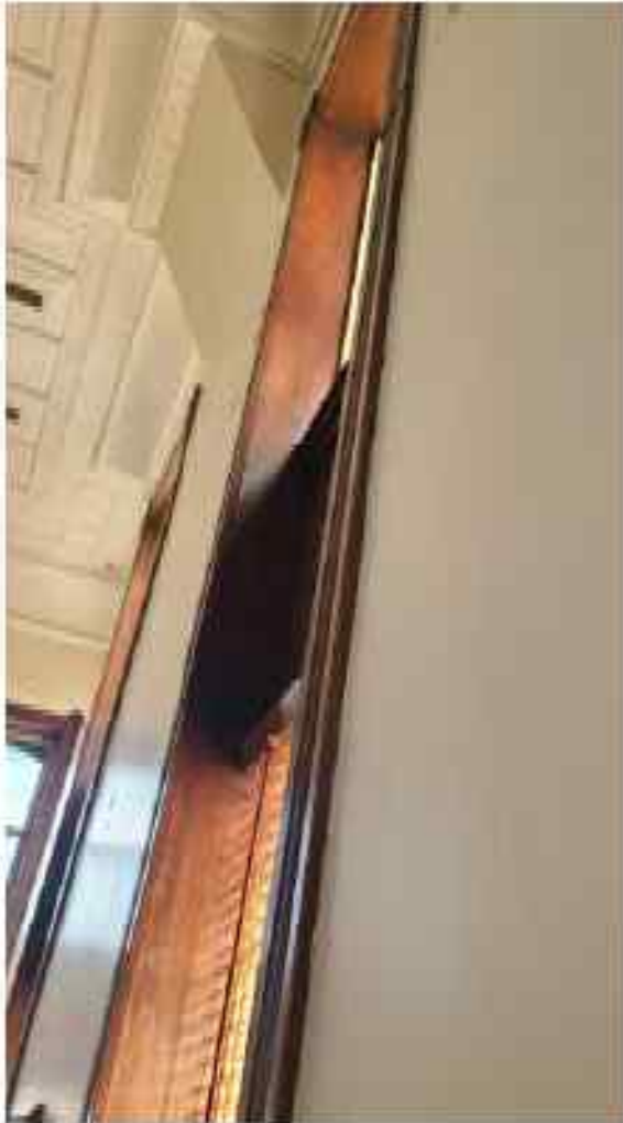
Image 56 - Typical wood deterioration at District Courtroom Windows
